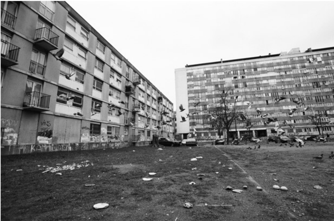
Fig. 2 - The use of cheap buildings materials caused physical degradation in a short span of time. Clichy-sous-Bois, 2000, http://softmorningcity.files.wordpress.com/2011/04/clichysous.jpg .
