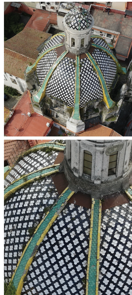
Fig. 4 - The extrados of the dome. Photo shooting from the drone. Survey by Mario Ronca, supervisor Manuela Piscitelli.
