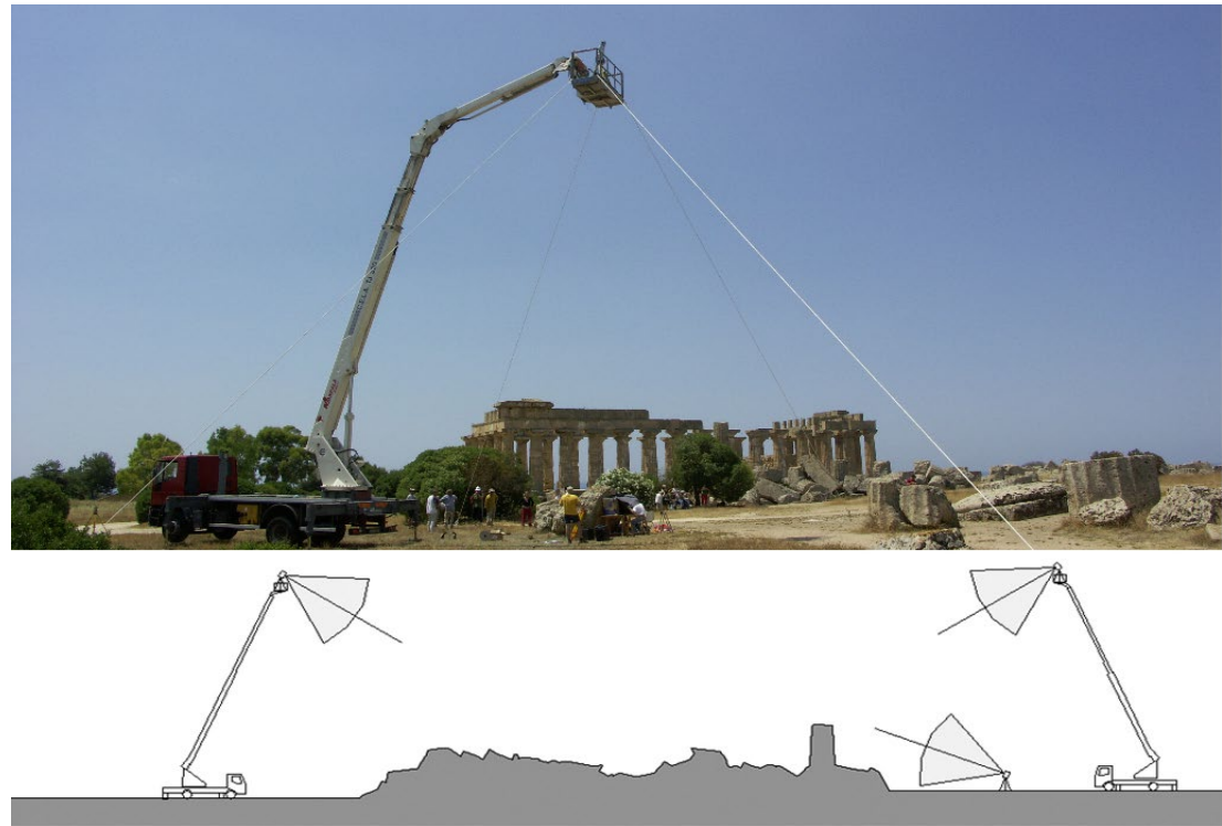
Fig. 4 - The mobile platform, stabilized with ropes, used in 2005 for the acquisition of laser scans.
