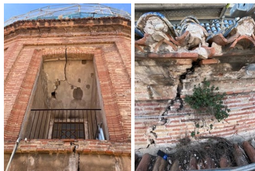
Fig. 2 - Cracks in the lintel and flare of the drum window (left) and in the second ring of the drum where it meets the roof (right).
