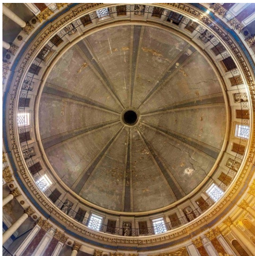
Fig. 1 - Interior view of the dome with the cracks.
