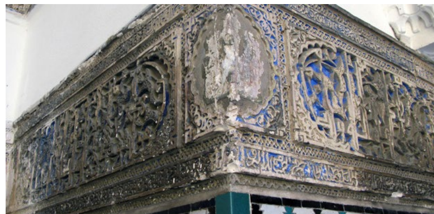
Fig. 2 - Pathologies in the plasterwork frieze of the Patio de las Doncellas (Campos de Alvear, 2020, p. 83)
