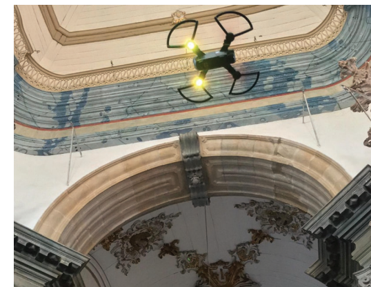
Fig.2 - Use of UAV for inspections and detailed acquisitions of outdoor and indoor environments. Image by P. Becherini, R. Volzone, A. Cottini, "A 3D model for architectural analysis, using aerial photogrammetry, for the digital documentation of the convent of Santa Maria da Insua, on the northern boarder between Portugal and Spain". (Proceedings of the 2nd D-Site conference).
