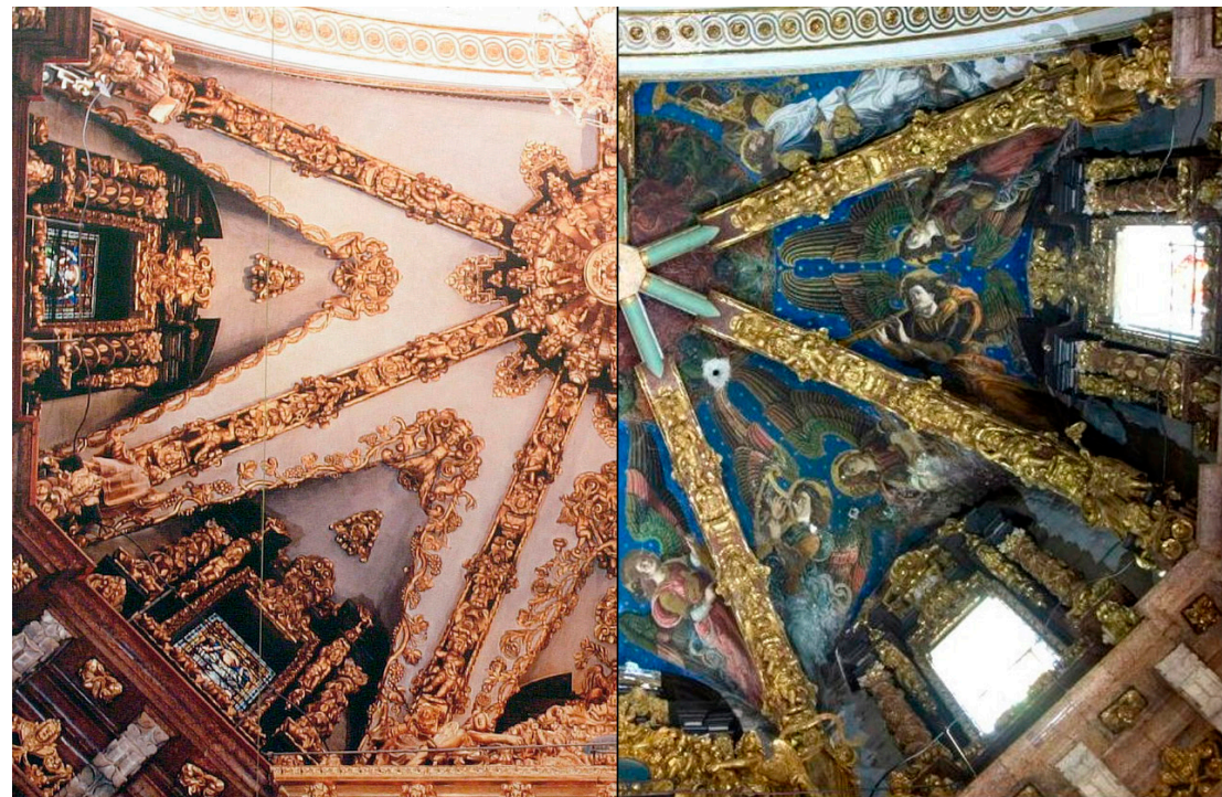
Fig. 1 - Photomontage of the state before (left) and the state after (right) the intervention to dismantle the baroque vault.
