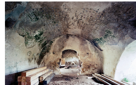
Fig. 13 - . Vaulted structure lightened and insulated with hollow bricks in a building of masseria Forgiano in Isola Capo Rizzuto (KR). Photograph by Alessandra Chemollo.
