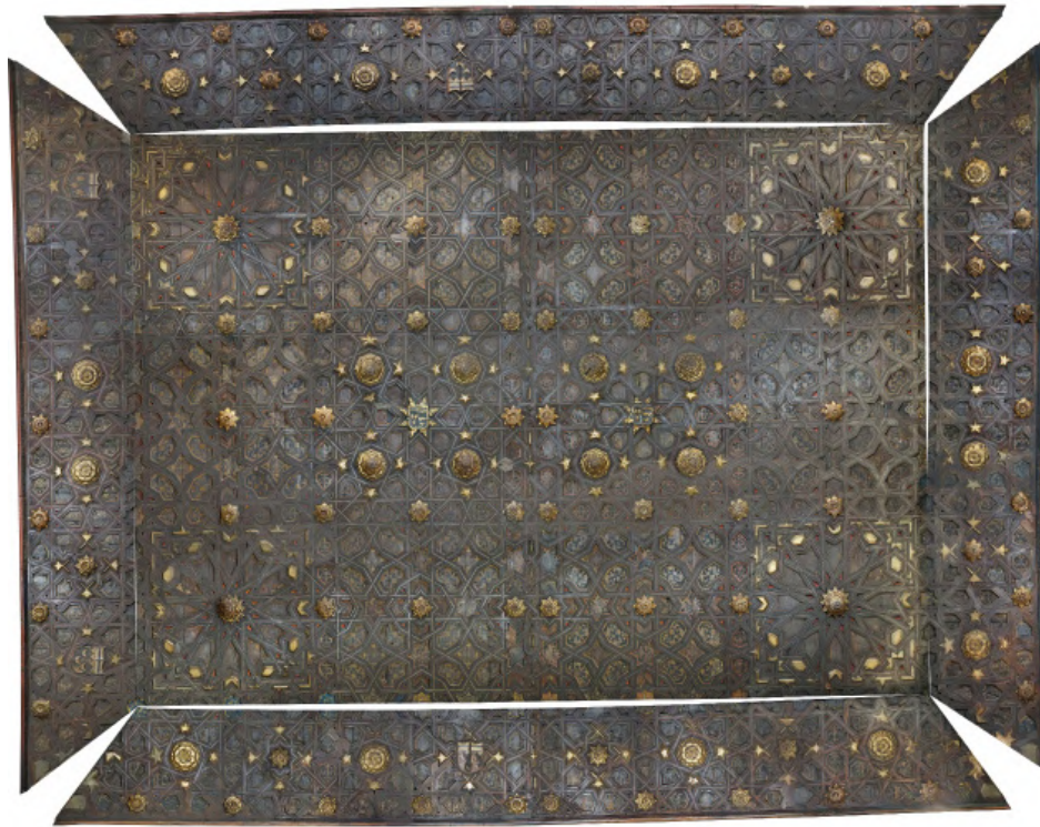
Fig. 15. Orthoimage of ceiling located in the mezzanine floor. Source: Reinoso, Gámiz & Barrero, 2021.
