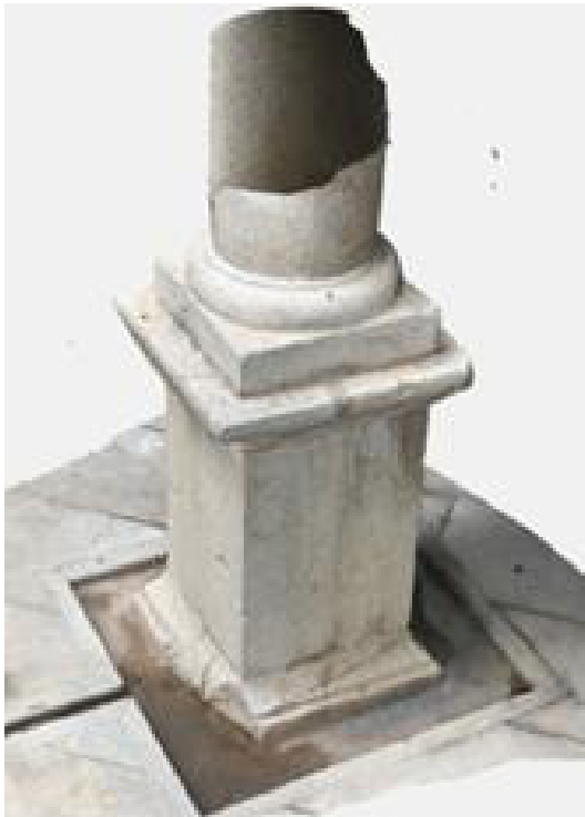
Fig. 6 - Column base produced by passive systems of Image of the convent of Dominicos in Castellón de la Plana, Spain.
