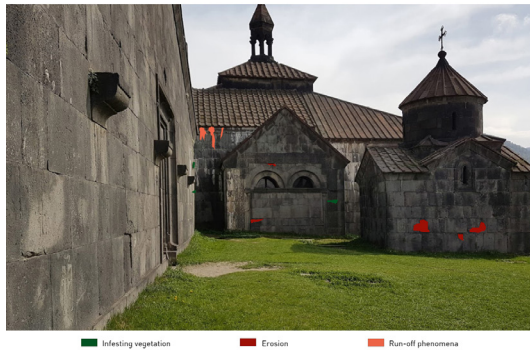
Fig. 9 - Monastery of Haghpot: state on conservation in April 2017 (above) and degradation form (bottom).
